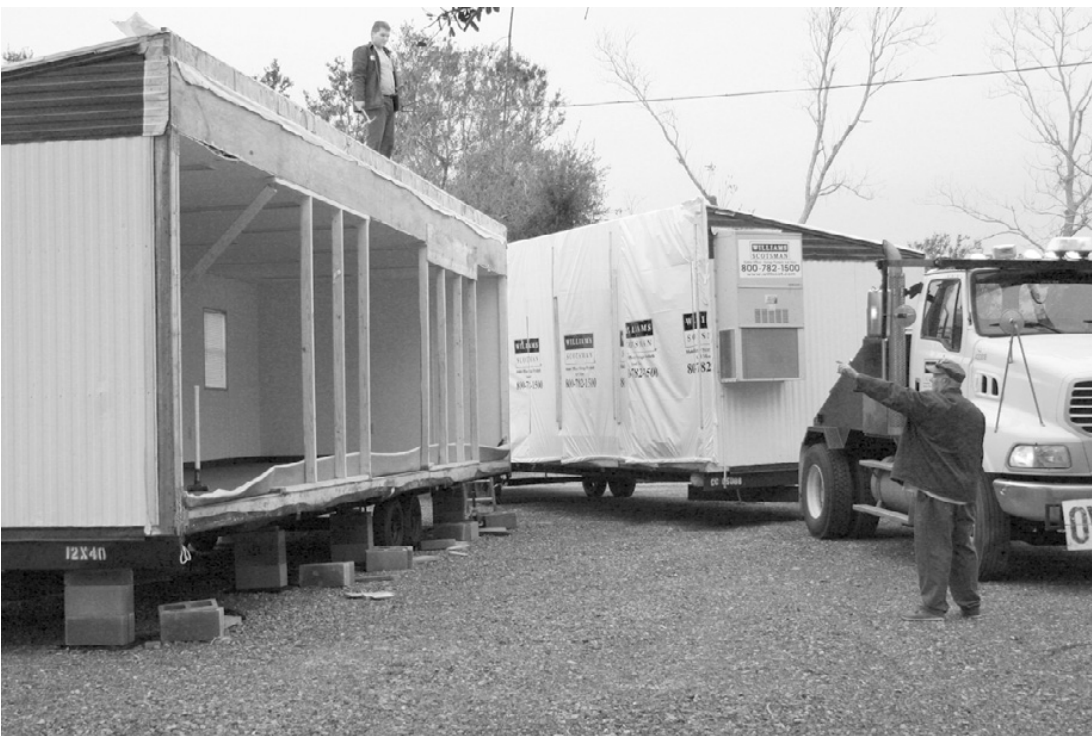
GRAND CHENIER'S temporary library building arrived last week and has been set up on the site of the former Bonsall Grocery, which was being remodeled into a library when Hurricane Rita hit. Both Cameron and Grand Chenier branches will be open within the next few weeks, thanks to a grant from the Gates Foundation, administered by SOLINET. (Photo by Cyndi Sellers.)
