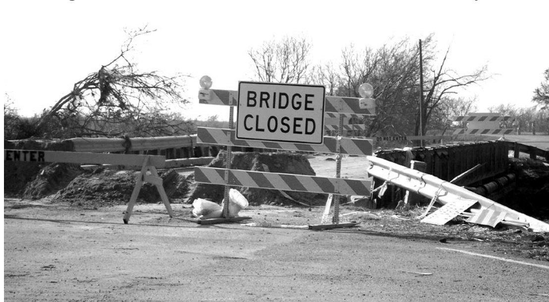
THE BRIDGE at Oak Grove is closed until repairs can be made in April or May, according to the Department of Transportation, and Development.
