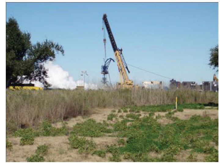
EFFORTS ARE continuing to cap a blowout gas well in the Oak Grove area. The well blew out on Jan. 6 but poses no danger to the area. Equipment is shown above attempting to shut off the well.
