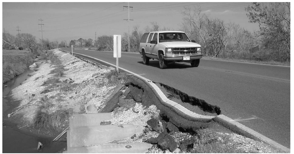
HWY. 27 between Creole and Cameron still has major damage to the road shoulders. The contractor is working south of Hackberry and in Grand Chenier. This section is scheduled to be repaired by May. (Photo by Cyndi Sellers.)
