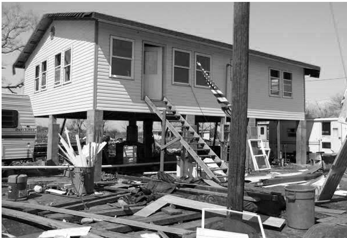
CAMERON COMEBACK - This new house in Phillips 66 subdivision is being built by Brian Debarge. He has been working on it for 22 days and expects to be finished next week. He said he can't wait to be out of his camper and into a real house. New building codes went into effect March 1, which may delay future housing.
