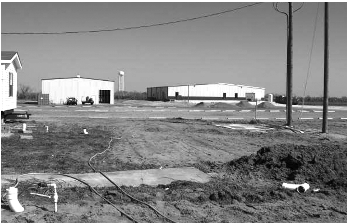
ROTORCRAFT LEASING has been working on this new heliport since before Hurricane Rita. They were back at it immediately after the storm, and the facility, located on Trosclair Road, is nearing completion. (Photo by Cyndi Sellers.)
