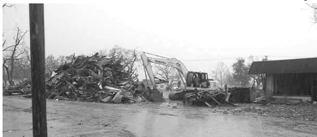
THE FORMER Dyson's Lumber Company building was razed last Saturday. The two-story building went through Hurricane Audrey, sheltering people on the second floor. When the water went down, several families found the upstairs a dry place to sleep until evacuation could take place the next day. Owned by former State Representative Alvin Dyson, the company was involved in rebuilding much of lower Cameron Parish after the storm. The passage of time and Hurricane Rita proved too much for the old building, however, and another Cameron landmark is gone.
