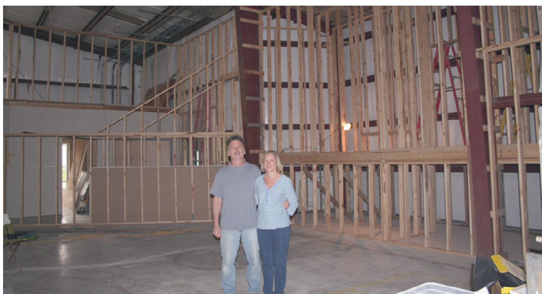
JOHN AND LINDA Doroshenko , of Bellingham, Washington, spent three weeks in Cameron framing the interior of the First Baptist Church sanctuary. The couple were on vacation from their house renovating business and located the church through a Bellingham company that sent a boat to the Sheriff's office after Hurricane Rita. It was their first time to volunteer, except for friends and family, but they enjoyed it so much they extended their stay an extra week. (Photo by Cyndi Sellers.)
