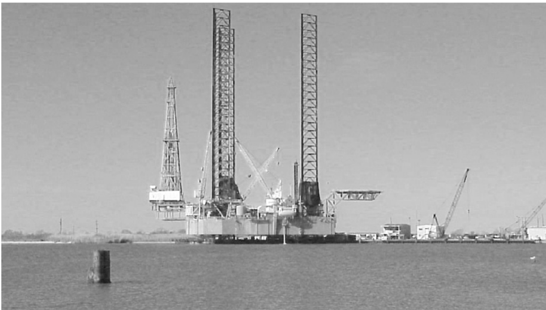
THE FIRST RIG TO come into Cameron under the new tax exemption ordinance is docked at TESORO (West) for refurbishing. A crew of over 100 workers from Port Arthur, Texas is expected to take 3-5 weeks to complete the project.
