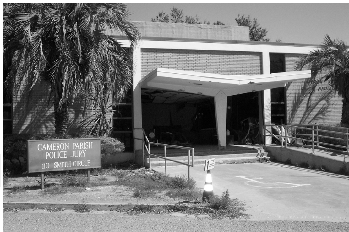
THE CAMERON PARISH Police Jury building was badly damaged by Hurricane Rita, although this view of the front fails to show it. The back of the building was caved in and the building was completely flooded. The building probably will be repaired some time in the future.
