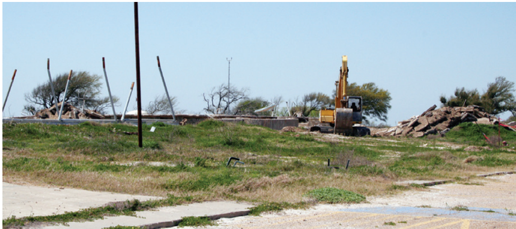
DEMOLITION IS under way at the Cameron Recreation Center. The remains of the pool are seen. The building is already gone, as are the tennis courts. (Photo by Cyndi Sellers.)
