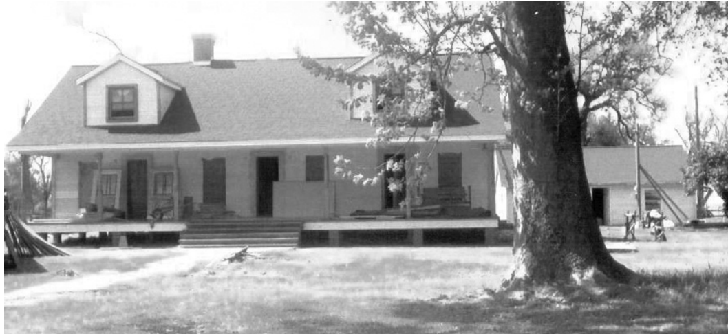
THE OLD VINCENT home in Hackberry, which was built in the 1860s, is being repaired and remodeled following roof damage in Hurricane Rita in 2005.
