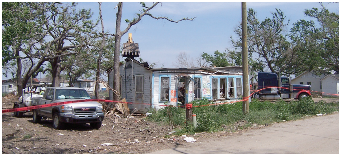
DEMOLITION OF private property began April 6 in Cameron Parish. This house behind the Cameron Courthouse was one of the first. Since it had asbestos products, at least 16 people were involved in the cleanup. (Photo by Cyndi Sellers.)
