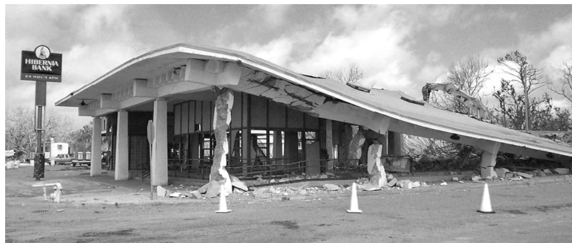
THE HIBERNIA Bank branch is being demolished, with great difficulty, to make way for a modular building expected to arrive this week to house bank services for Cameron residents. The old building's supports and roof were made of reinforced concrete, built to withstand hurricanes. Demolition began last Saturday. (Photo by Cyndi Sellers.)
