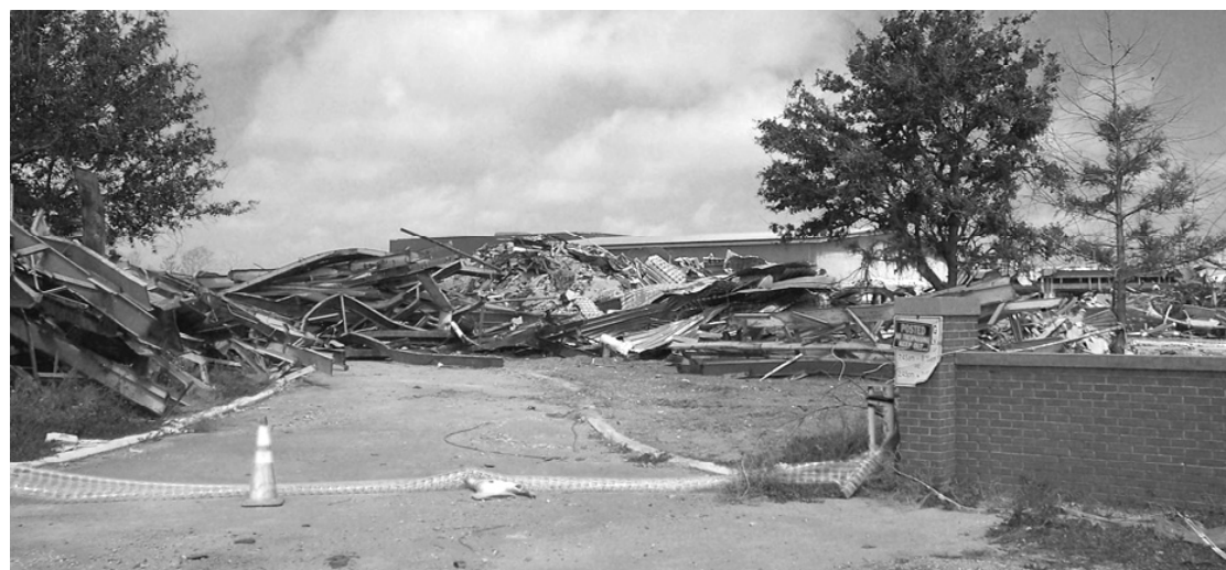
DEMOLITION continues at South Cameron High School in Creole. Most of the building is being removed to make way for a K - 12 school for students from Cameron, Creole and Grand Chenier. The gyms are being saved for use while the school is located in modular classrooms this fall. (Photo by Cyndi Sellers.)
