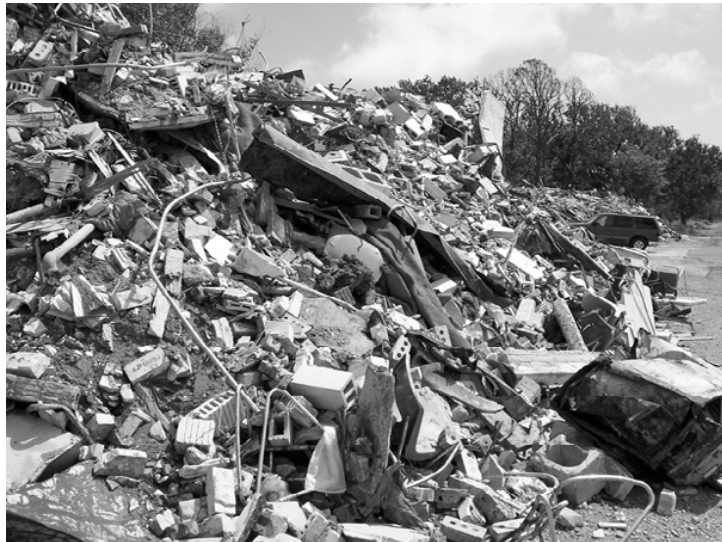
PILES OF DEBRIS have accumulated as the South Cameron High School is demolished to make way for a K - 12 school. (Photo by Cyndi Sellers.)
