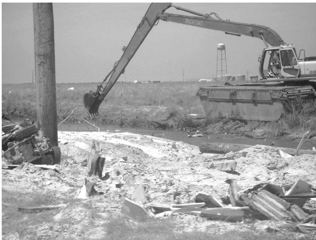
TIS LARGE machine is shown cleaning debris out of roadside ditches at Holly Beach. this coastal community was wiped out by Hurricane Rita but some mobile homes are being moved in. (Photo by Cyndi Sellers)
