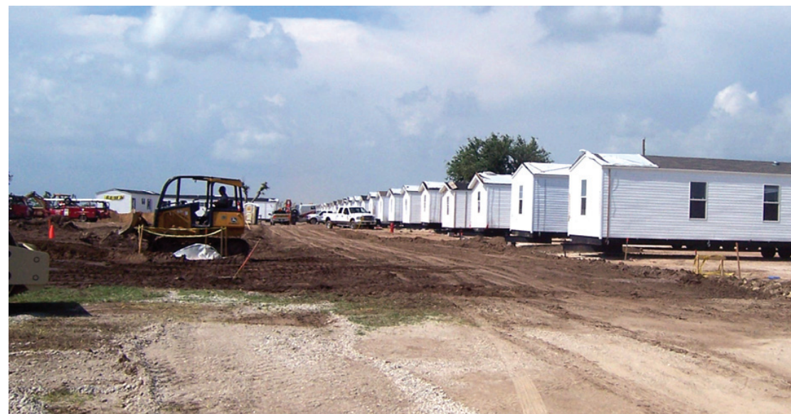
THIS FEMA MOBILE home park being constructed in Grand Lake is causing some distress for neighbors, who have requested a 6' wooden privacy fence be erected around it. The park has 38 displaced Cameron Parish families signed up so far, and will house 60 families when complete. (Photo by Cyndi Sellers.)
