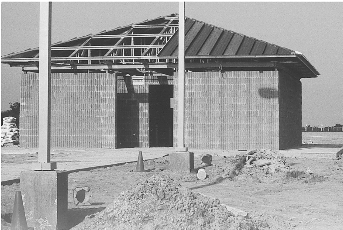
NEW RESTROOM facilities are being built at the Jetty Pier Park at Cameron. The $169,700 project was paid for by a grant from the Governor's Office of Rural Development. Sam Istre Construction Company is the contractor. The park is administered by the Cameron Parish Police Jury. (Photo by Cyndi Sellers.)
