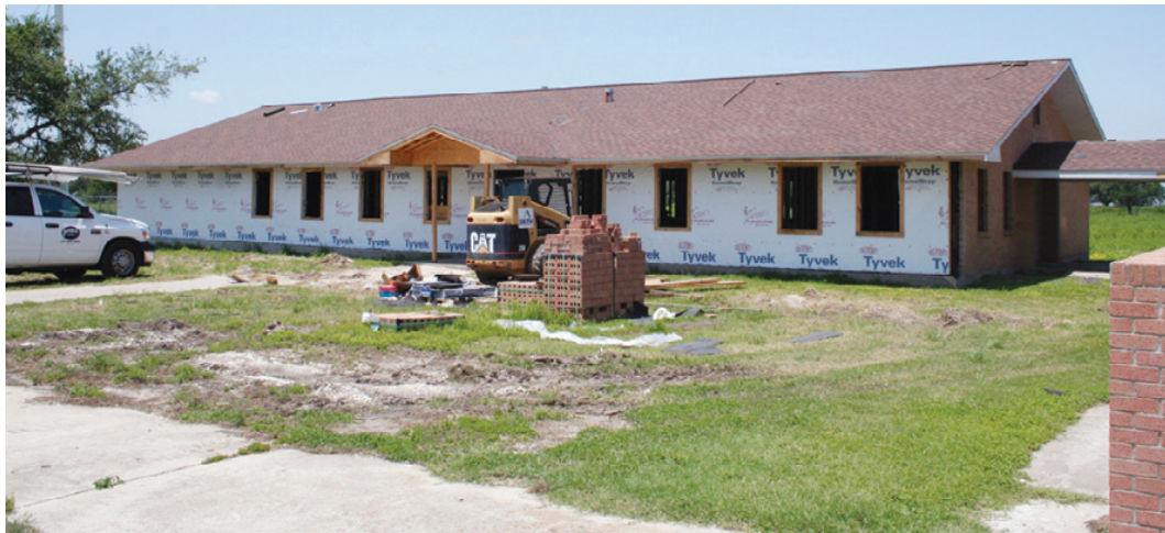
WORK HAS BEGUN on the church hall and rectory at St. Eugene Catholic Church in Grand Chenier. Funds for the remodeling have been raised by the congregation through the annual Alligator Festival and other fundraisers.
