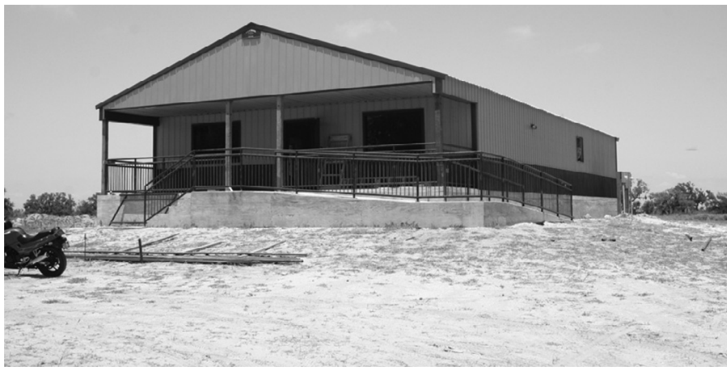
BOOTH'S GROCERY in Grand Chenier is nearing completion. Mrs. T-Mae Booth vowed to rebuild after Hurricane Rita and plans to live in the back of the store when complete, sometime later in the summer. (Photo by Cyndi Sellers.)
