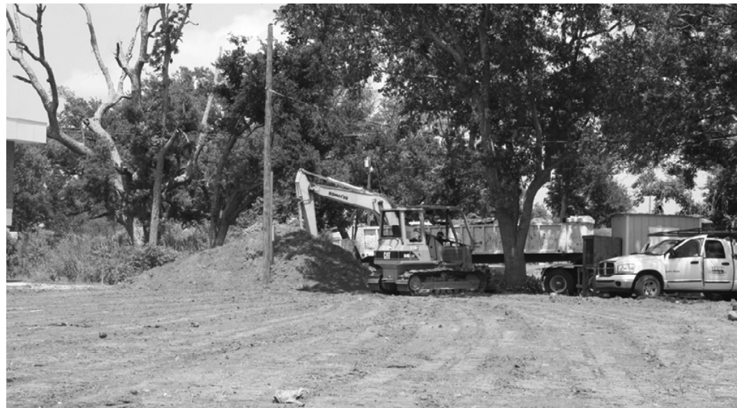
WORK HAS finally begun on the East Annex on Courthouse Square in Cameron. Lewing Construction started dirt work at the site of the former Police Jury Annex on Tuesday. The bid was approved on April 7. (Photo by Cyndi Sellers.)
