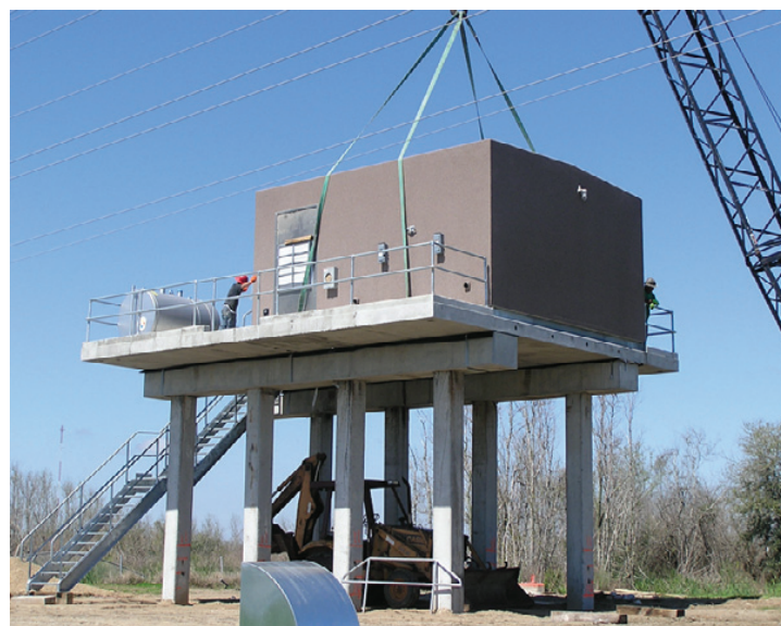
CAMERON COMMUNICATIONS has completed the rebuilding of its central offices at Creole, Grand Chenier, and Johnson Bayou which were destroyed by Hurricane Rita. The Johnson Bayou office is shown above.
