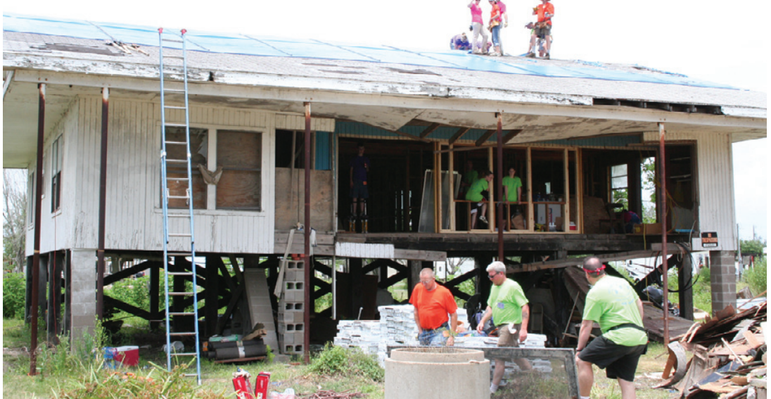
TWENTY EIGHT volunteers from the Eight Days of Hope disaster relief organization work on Peggy and Oscar Reyes house in Cameron. The team is gutting, re-roofing, rewiring, installing new supports and windows, and as much more as they can by the end of the week. (Photo by Cyndi Sellers.)
