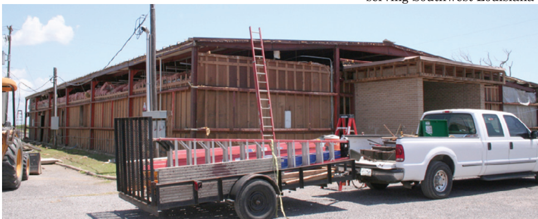
WORK HAS BEGUN on repairing the Cameron Multi-Purpose Building, site of the Fur and Wildlife Festival in former years. The building was left mostly intact by Hurricane Rita, but was used for various storage purposes after the storm instead of being repaired. It housed caskets and remains from area cemeteries, then fire trucks, and finally miscellaneous items until a FEMA project worksheet was completed. (Photo by Cyndi Sellers.)
