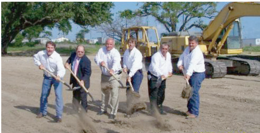
PICTURED ABOVE are the Cameron Parish Police Jurors breaking ground for the East Annex Building in Cameron Square. The architect for the new building is Randy Goodloe and the Contractor is Lewing Construction. The former building was destroyed by Hurricane Rita.
