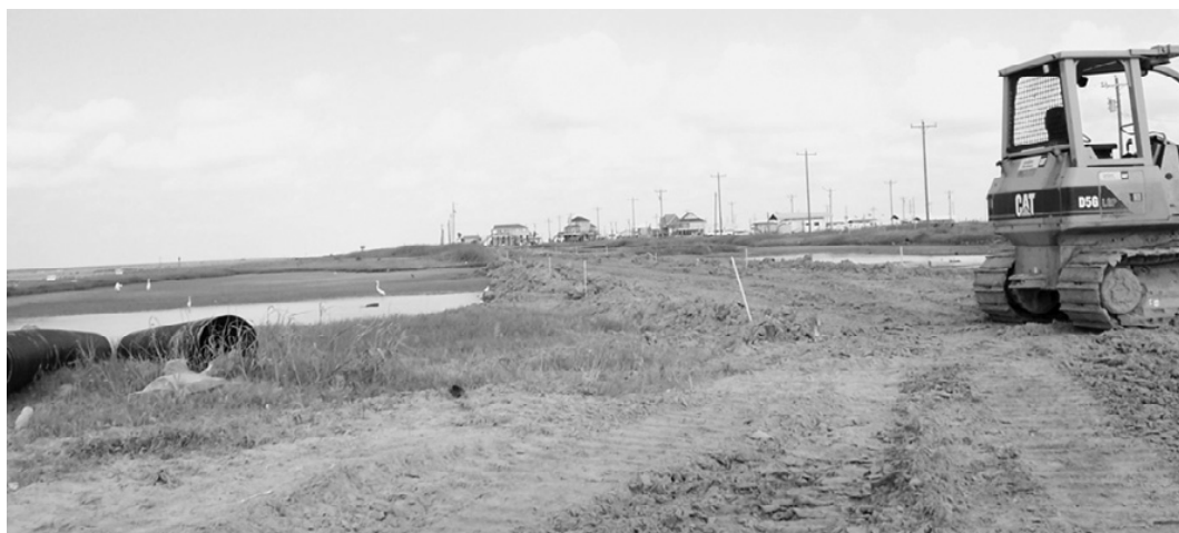
PARISH ROAD 512 in Holly Beach, popular with beachgoers for many years, is being restored. A large scour pit had claimed part of the road during Hurricane Rita. Last week crews pumped out the pond and extended the road through it. The sides will be reinforced with rock to protect against future scouring.
