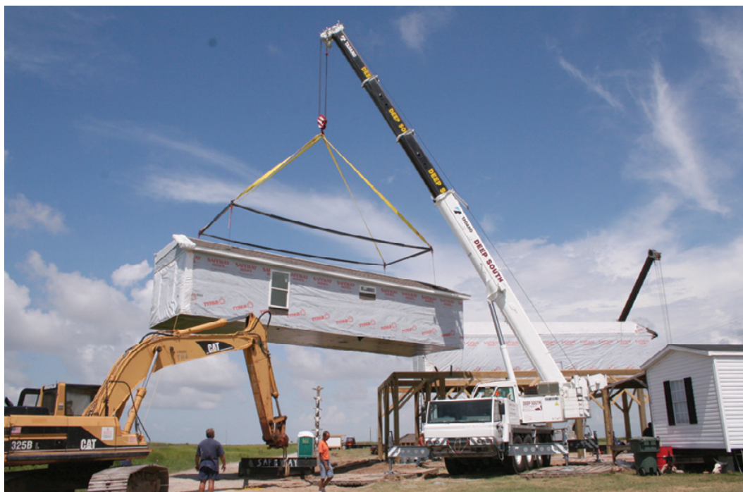
THE FIRST HOUSE to be built at Rutherford Beach since Hurricane Rita was assembled Tuesday. It belongs to Roman Theriot. The modular home is built to withstand 150 mph winds. Contractor Rick Hagel, of Pintail Construction and Development, said this method cuts construction time almost in half as compared with a traditional stick framed house, and at a lower cost. The three modules were built off site and were connected once they were in place on the foundation.
