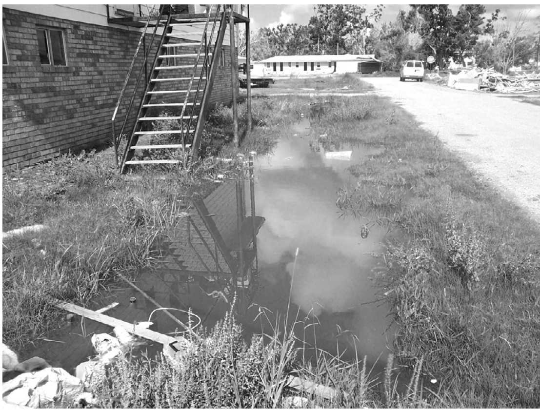
HEAVY RAINS on Monday have left standing water in many ditches and yards around Cameron. The culverts are plugged with storm debris and mud and the stagnant water is beginning to smell and breed mosquitos. (Photo by Cyndi Sellers.)
