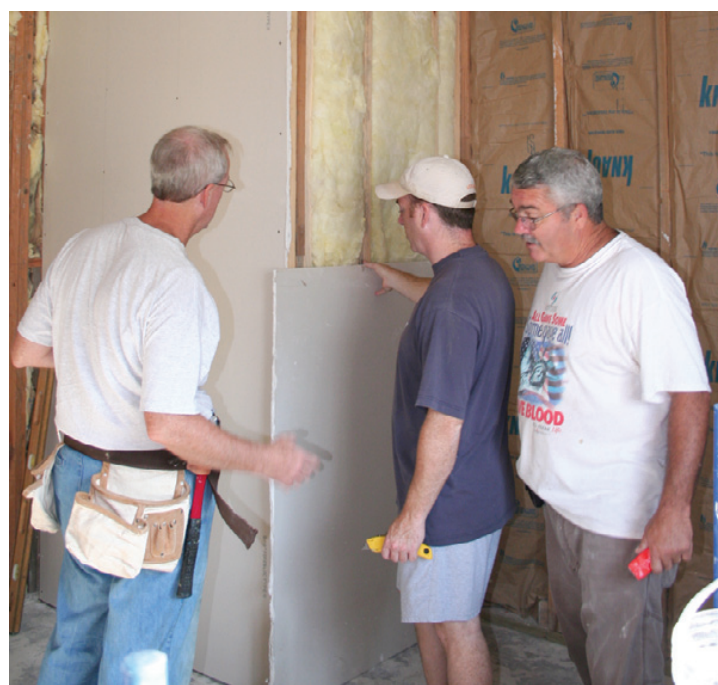
MEN FROM Northstar Baptist Church in Bristol, Tenn., worked at the First Baptist Church in Cameron last week, hanging sheetrock in the church kitchen and restrooms. FBC hopes to have the fellowship hall ready for use by the end of the summer. Work on the sanctuary will begin soon. (Photo by Cyndi Sellers.)
