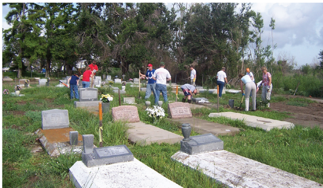
YOUTH FROM Northstar Baptist Church in Bristol, Tenn., helped clean the First Baptist Church cemetery near Cameron last week, even though it rained nearly every day. The group also worked to repair the church. (Photo by Cyndi Sellers.)
