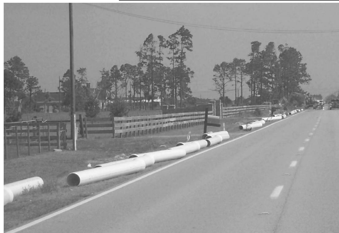
PIPE FOR WATER badly needed by the Grand Lake community is being laid south from the Lake Charles airport. (Photo by Cyndi Sellers.)
