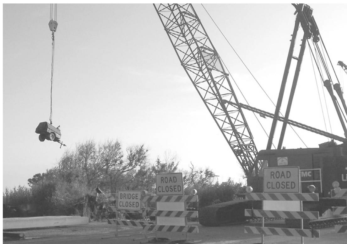
AN INTERESTING way to protect equipment from theft - seen at the site of the bridge repair in Oak Grove. (Photo by Cyndi Sellers.)
