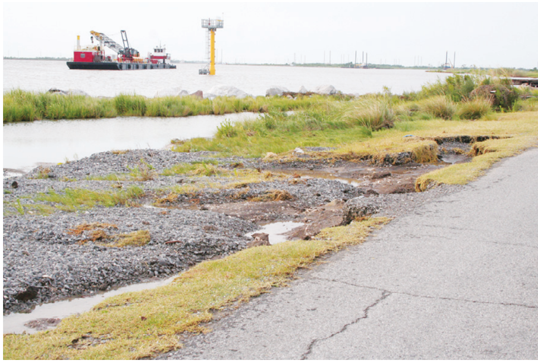
MINOR SHOULDER damages occurred when water ran across David Road near the Cameron jetties on Tuesday during Tropical Storm Edouard. (Photo by Cyndi Sellers.)
