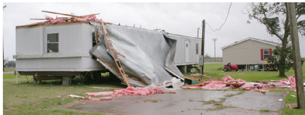
THREE MOBILE homes on Hayes Picou Road in Cameron were damaged by Tropical Storm Edouard Tuesday morning. This one had its roof torn off. Another one lost a canopy and the third one had roof damage. A barn was blown down in Creole and a shrimp boat sank in Cameron. (Photo by Cyndi Sellers.)
