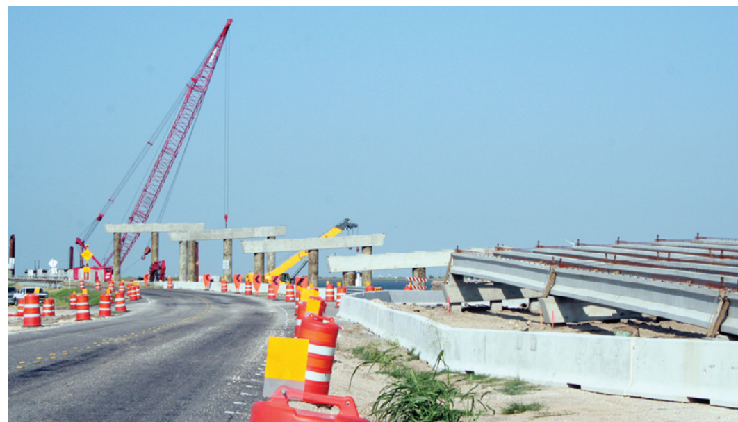
CONSTRUCTION OF the new Sabine River bridge, linking Cameron Parish with Pleasure Island in Texas, is progressing. This view is from the Texas side. (Photo by Cyndi Sellers.)
