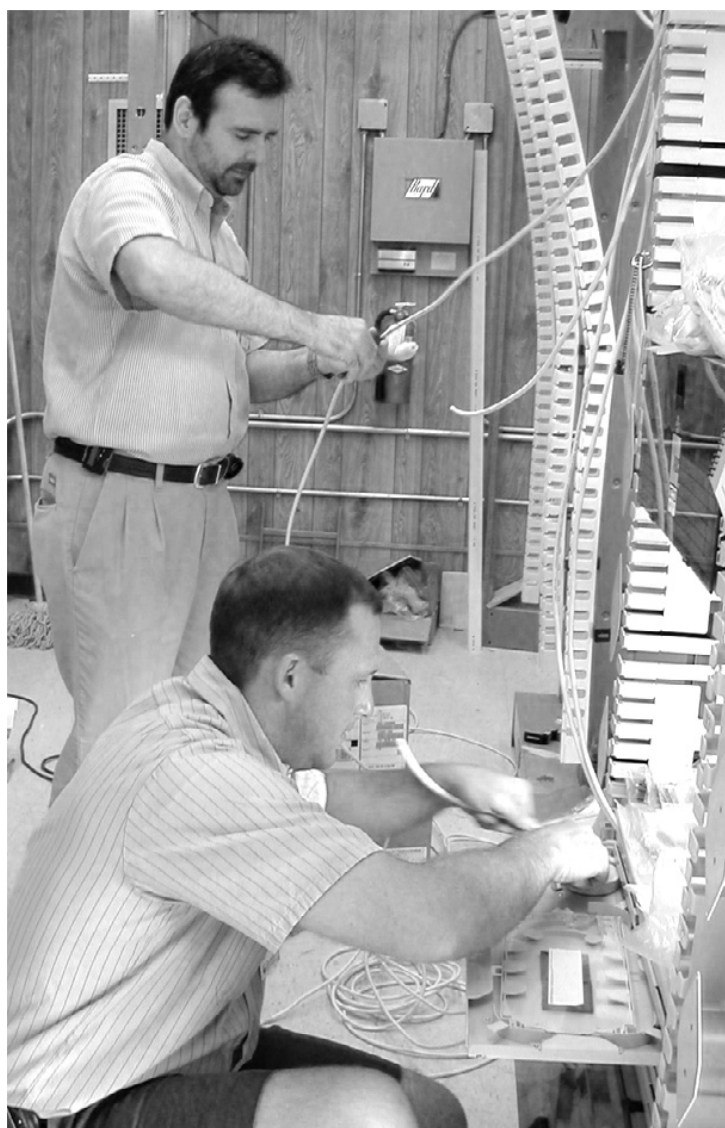
AT THE NEW Cameron Communications Grand Lake Central Office, Howard Latiolais, Chief Engineer, and Chris Cormier, Fiber Technician, prepare fiber tip cables and connector panels for splicing to the outside buried fiber optic line for the Grand Lake Fiber-to-the-Home project. Fiber optic cables link the connector panels to send digital voice, data and video to the Grand Lake community beginning this fall. FTTH will feature ultra fast Internet access with speeds up to 3.0 Mbps, digital television with over 150 channels including all the area favorites, and telephone services with local calling to Lake Charles and all of Cameron Parish.
