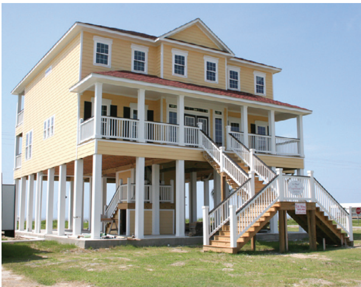
"LE PHARE - La Lumiere Apres L'Orage" (The Lighthouse - The Light After the Storm), is the name of this new beach house under construction at Holly Beach. It is one of several large residences beginning to replace some of the lost structures in the resort community. (Photo by Cyndi Sellers.)
