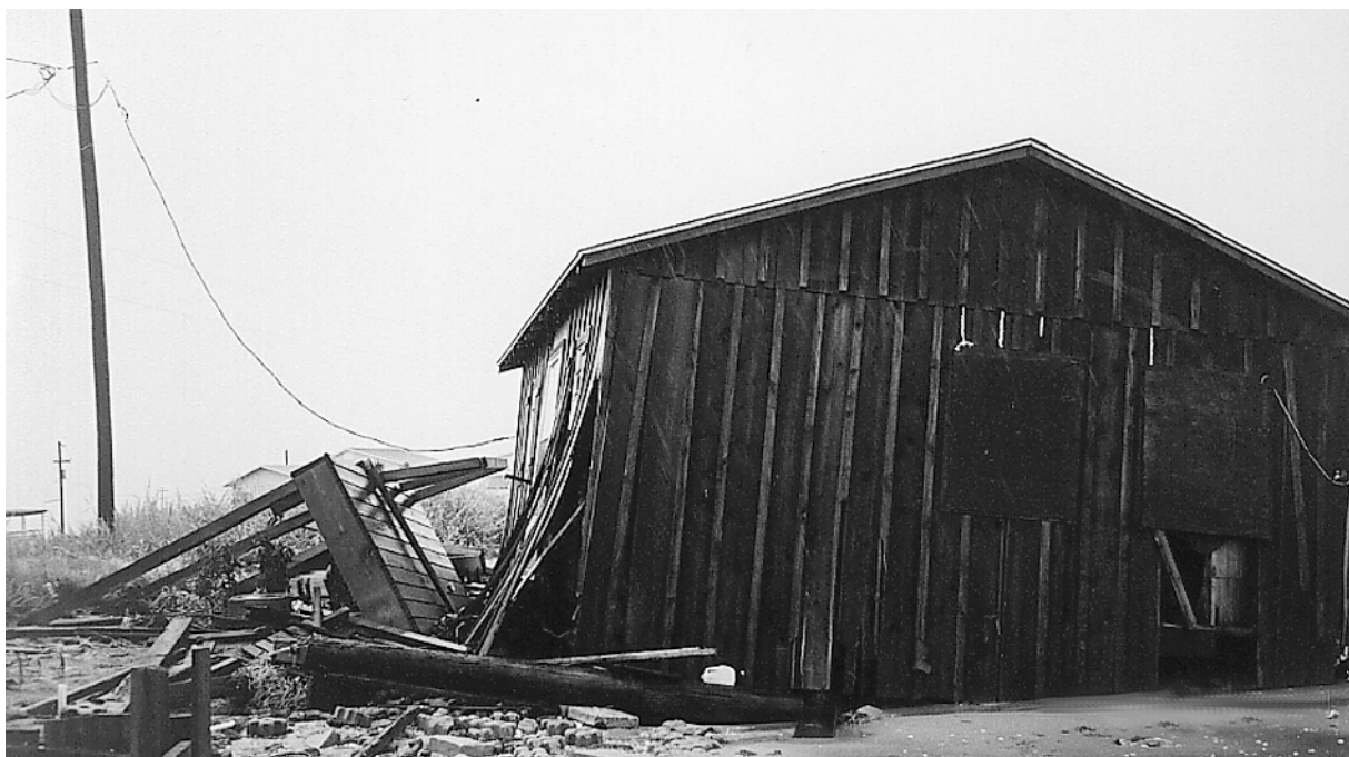
CONSTANCE BEACH again suffered significant beach erosion in the storm that hit on Aug. 8. This home on Richard Lane collapsed when the high tides undermined its foundation. This area of the coast has suffered extreme erosion in recent years. It is hoped by local residents that a project underway to pump sand in behind the breakwaters will protect beach homes. (Photo by Rodney Guilbeaux.)
