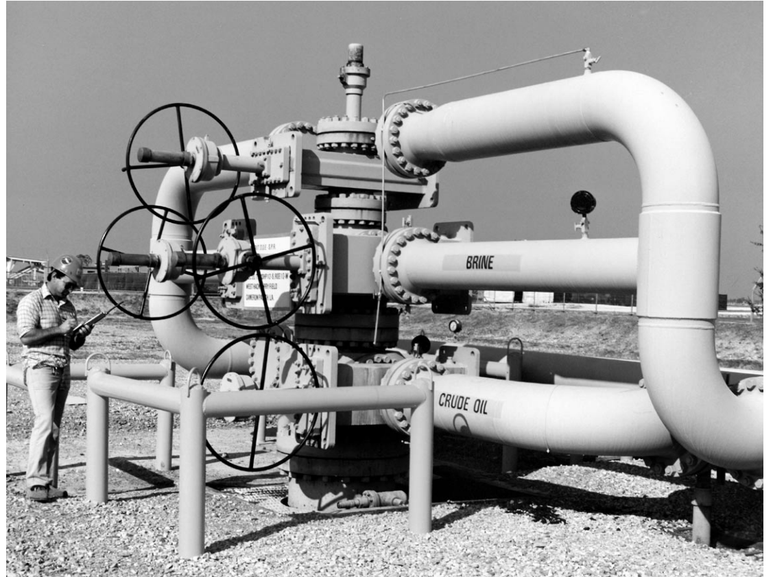
A TECHNICIAN is shown inspecting a wellhead assembly at the West Hackberry Strategic Petroleum Reserve site at Hackberry. Oil from this site may be among that being released this week on orders from President Bush to help with the crisis in the oil production industry caused by Hurricane Katrina.
