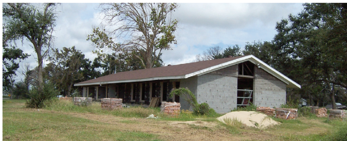
WORK HAS BEGUN on repairs to the Grand Chenier Methodist Church. Plans are being made to rebuild Wakefield Methodist Church in Cameron, as well, according to Rev. Wayne Taylor.
