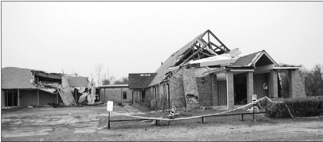
The damage done to St. Peter the Apostle Church in Hackberry is seen some two weeks following Hurricane Rita. The parish is still celebrating Mass in the damaged parish hall. Repairs to the religious education building and parish hall await completion of the church.
