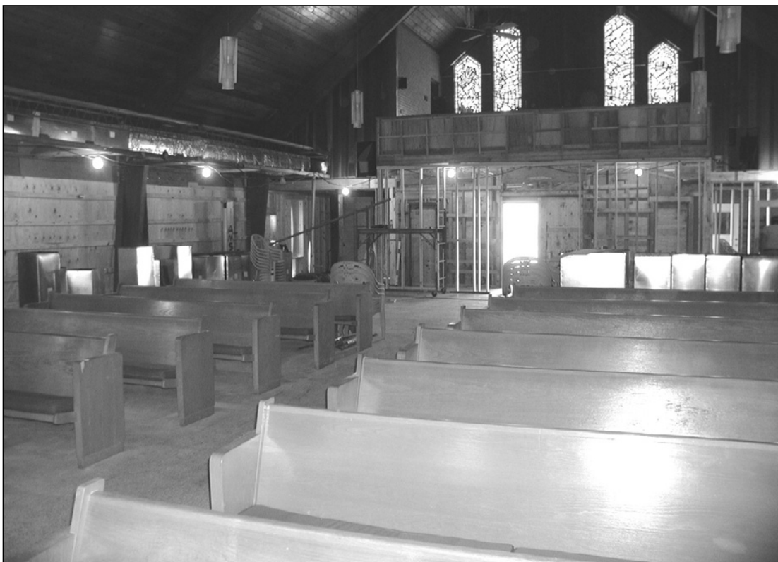
Work has begun on the church at St. Eugene. Much work remains to be done both inside and outside before the church can safely be used to celebrate Liturgy.
