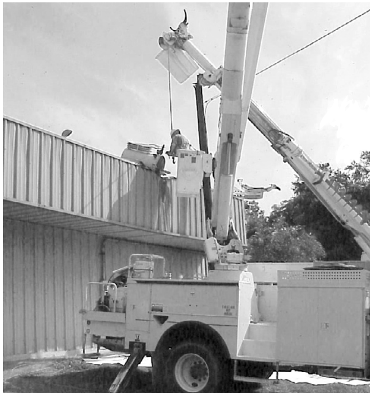
JEFF DAVIS Electric Co-op workers needed several hours to repair a utility pole that broke Saturday morning, dropping a transformer on the roof of 7X Square in Creole. Owner Ben Rutherford did not know how much it would cost to repair the roof. (Photo by Cyndi Sellers.)
