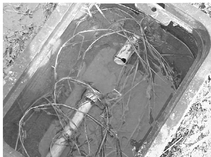
VANDALS CUT this water pipe leading to the picnic area at Rutherford Beach, preventing the Beach Sweep volunteers from having access to water. Vandalism is a recurring problem at the beach.
