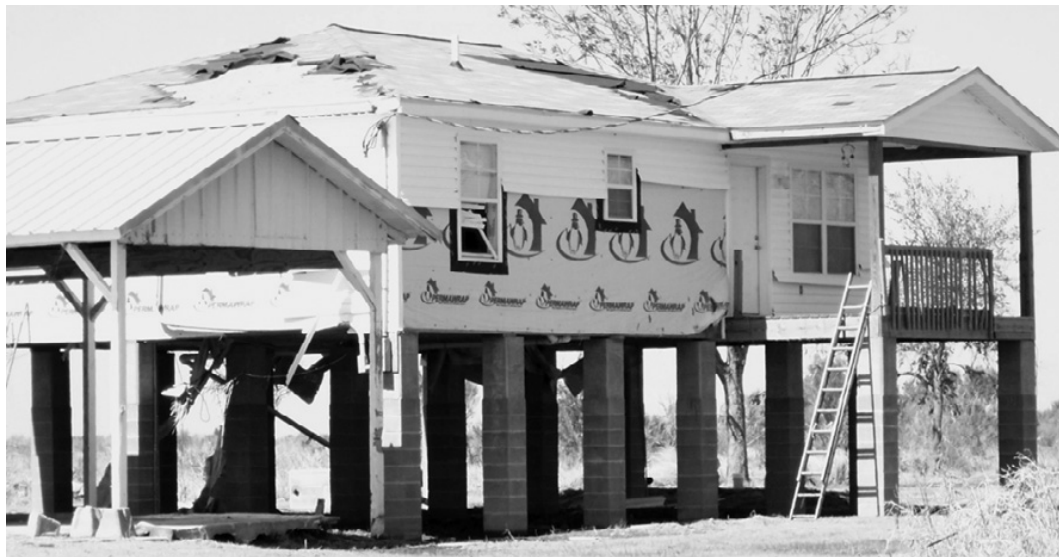
LEROY BLANCHARD'S home in Johnson Bayou sustained some damage, but is still standing. It was one of the homes built by the Mennonite Disaster Services and was dedicated in March of 2008. (Photo by Cyndi Sellers.)
