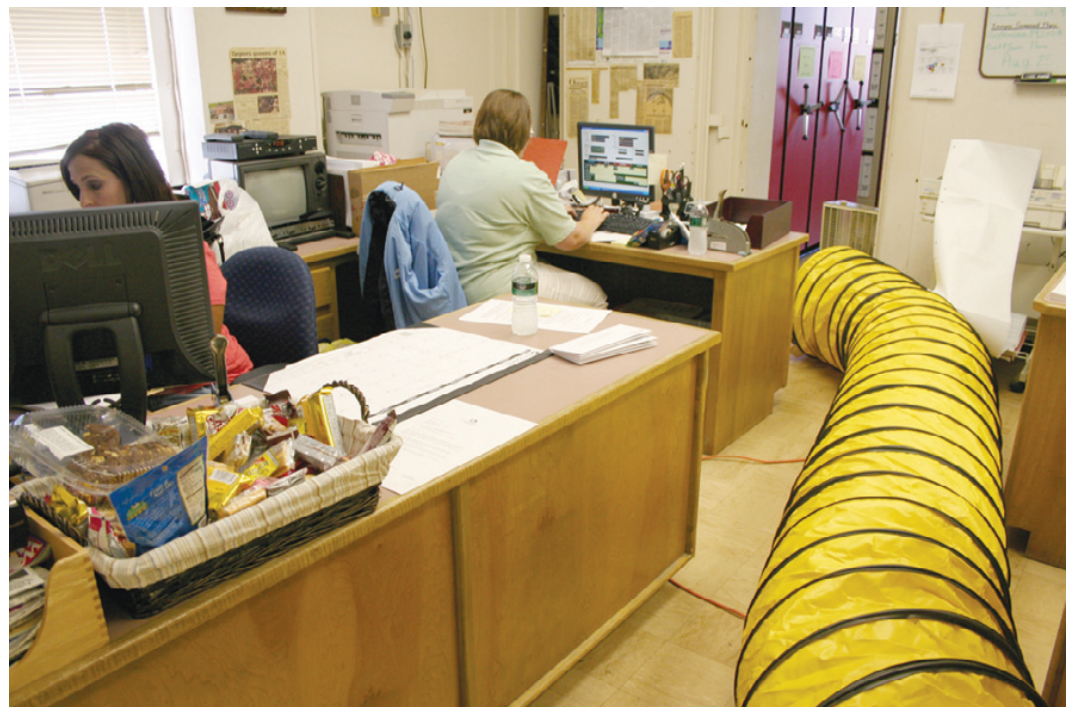
THERE'S ROOM for one person to walk through the Clerk's office past the giant air conditioning ductwork. (Photo by Cyndi Sellers.)
