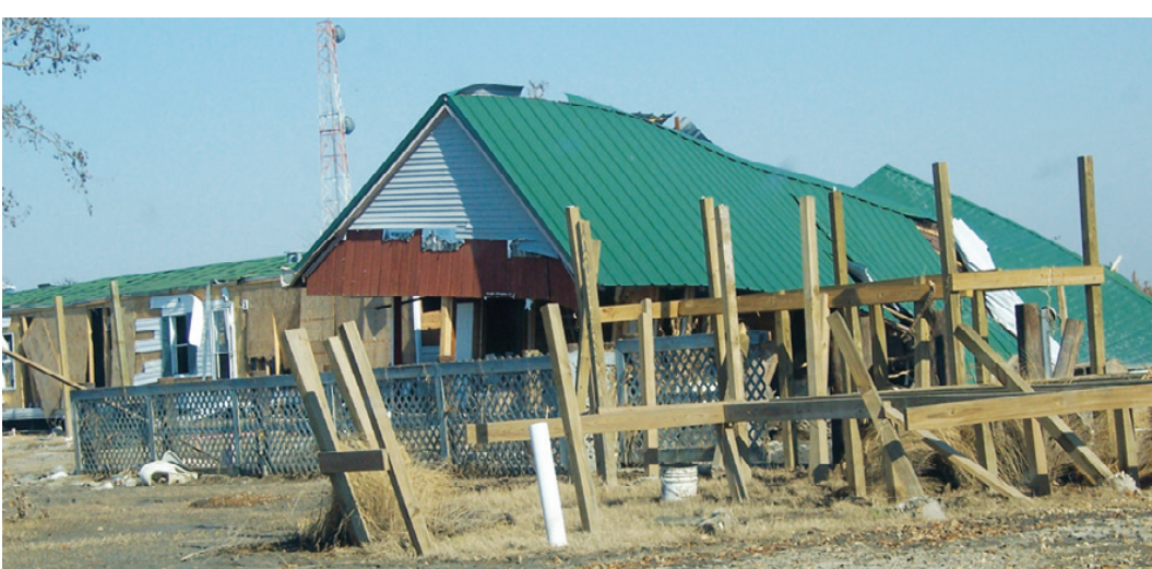
THIS HOUSE on Willow Lane off Smith Ridge in Johnson Bayou was knocked off its pilings. (Photo by Paul Sellers.)
