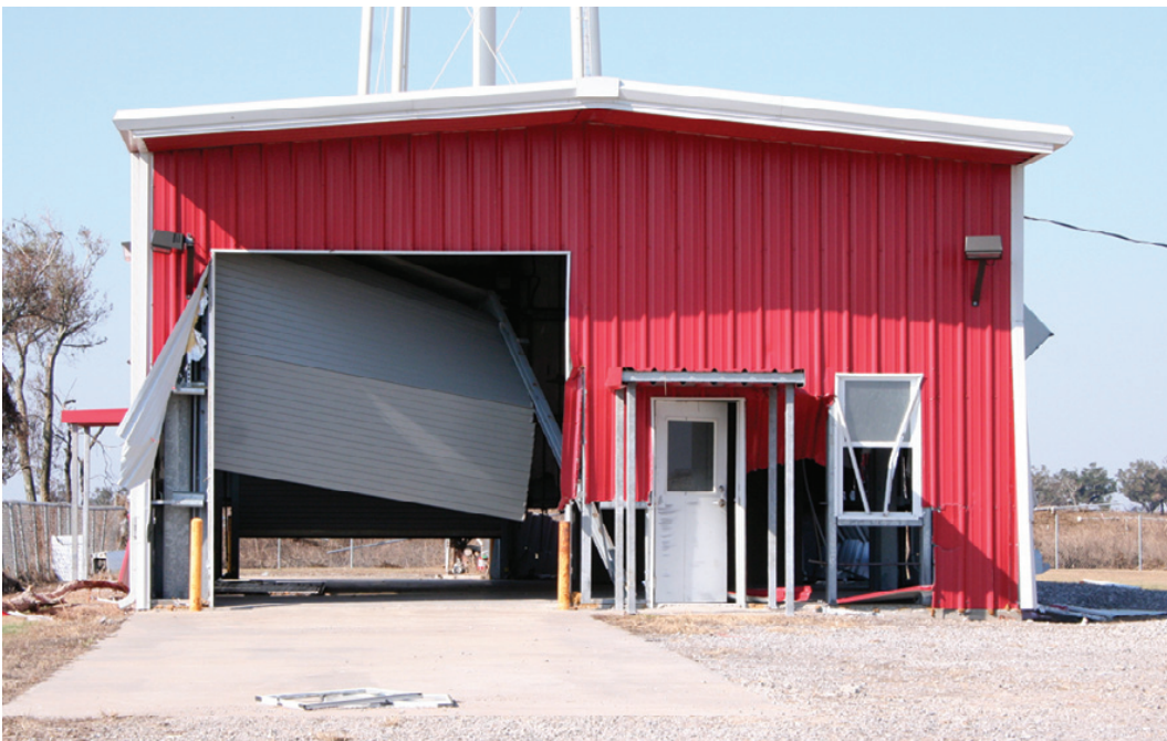
THE FIRE STATION at Grand Chenier sustained damage from Hurricane Ike. (Photo by Cyndi Sellers.)
