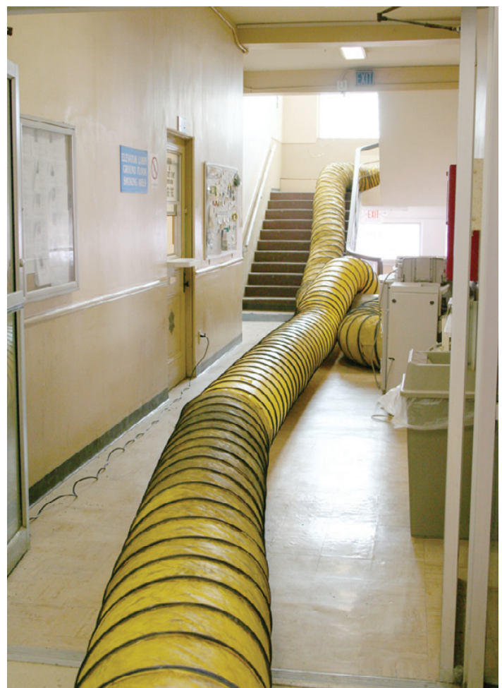
AIR CONDITIONING ductwork runs throughout the courthouse. (Photo by Cyndi Sellers.)
