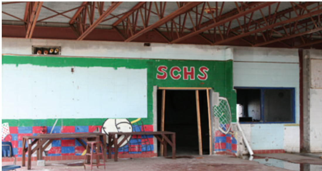
The "new" gym at South Cameron High School sits empty and un-repaired since the storm. A bid package is being prepared for repair options, but it will be at least 80 days before it can be used. Meanwhile, basketball teams are practicing in Grand Lake. (Photo by Cyndi Sellers.)
