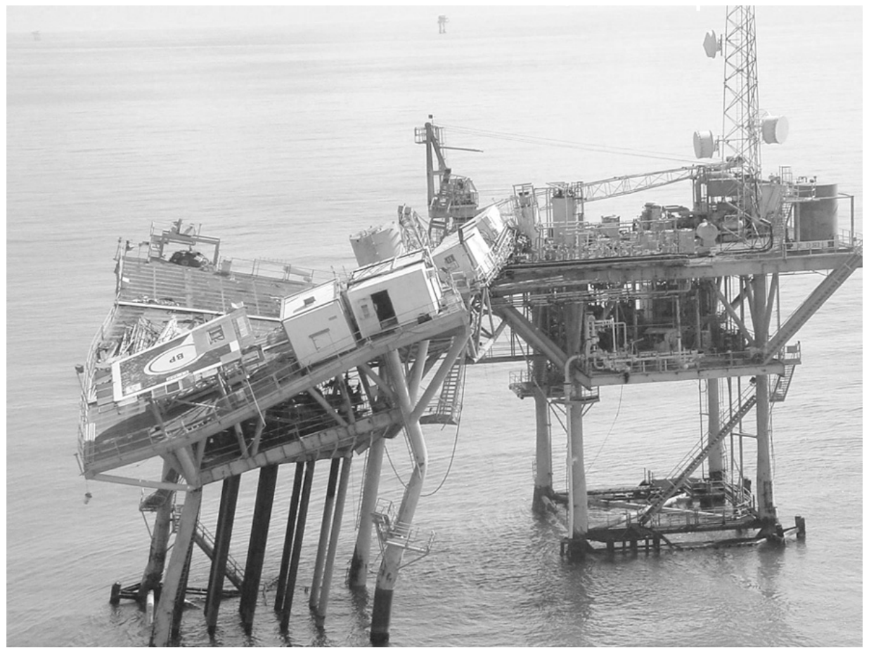
THIS IS A picture of a British Petroleum offshore platform that was destroyed by Hurricane Lili two weeks ago. The company reportedly lost two platforms in the storm. The exact location of this platform was not known.
