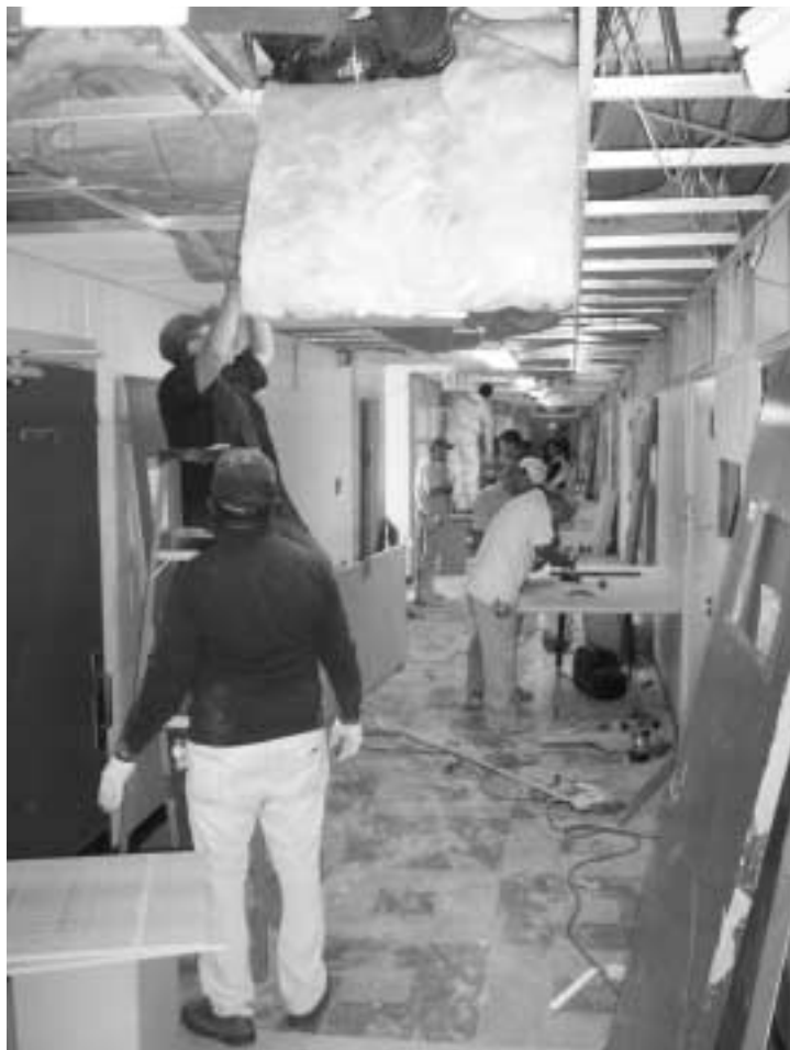
WORKMEN ARE shown busily getting Grand Lake High School in shape for opening on Thursday, Oct. 27. Hackberry High School will also open on that date. Cameron Elementary and South Cameron Elementary and High School students will also report to Grand Lake. Johnson Bayou students will report to Hackberry. The four schools in lower Cameron Parish were destroyed by Hurricane Rita.
