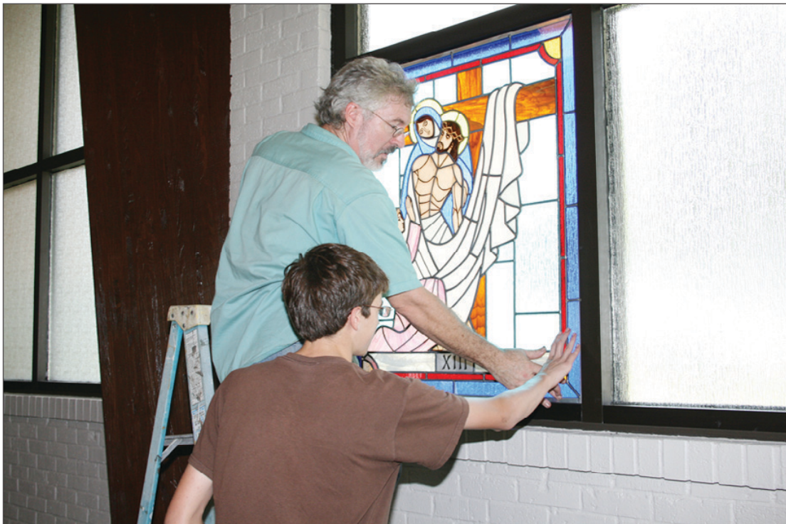
Frank Thompson, left, and his son, Levi, install one of the 14 Stations of the Cross in Our Lady Star of the Sea Church in Cameron. Here they put the finishing touches on the 13th Station – Jesus is taken down from the Cross.
