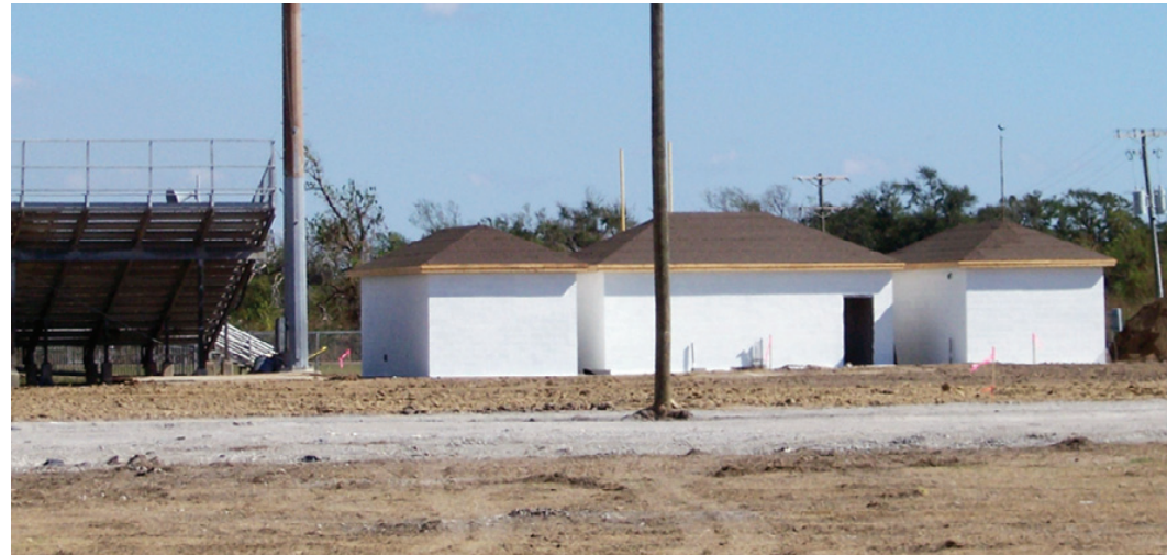
THE REST ROOMS and concession stand at South Cameron High School stadium are nearly complete. The school was destroyed by Hurricane Ike but will be rebuilt. (Photo by Cyndi Sellers.)
