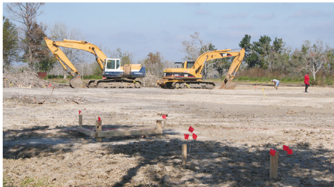
THE FOUNDATION IS being prepared for the new South Cameron Memorial Hospital. The Lower Cameron Hospital Service District has received the first $1.2 million installment of $16 million in FEMA funds allocated to rebuild the hospital.
