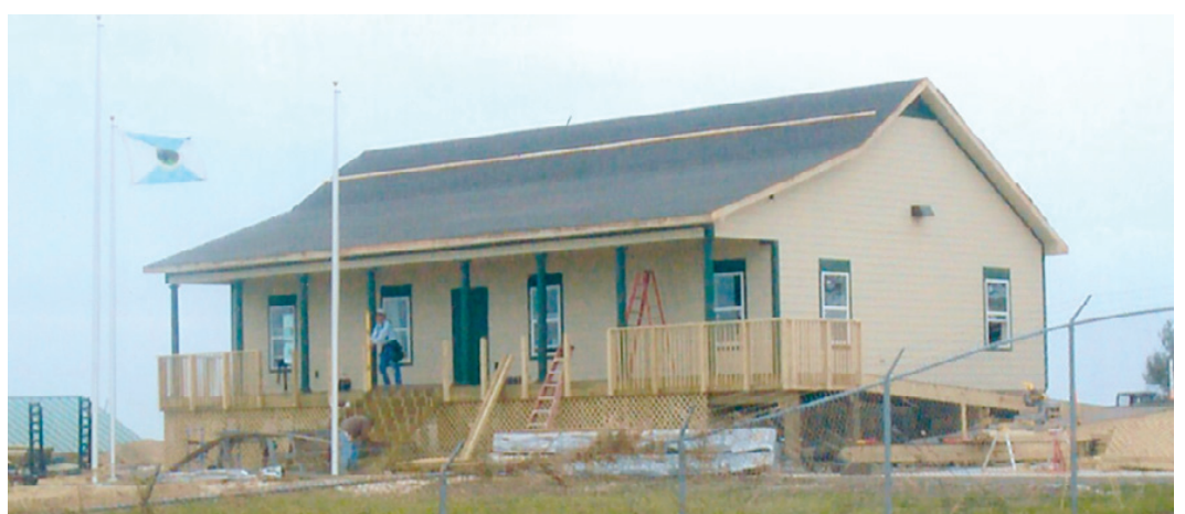
THE SABINE REFUGE headquarters building is now under construction. The refuge buildings were destroyed by Hurricane Ike.
