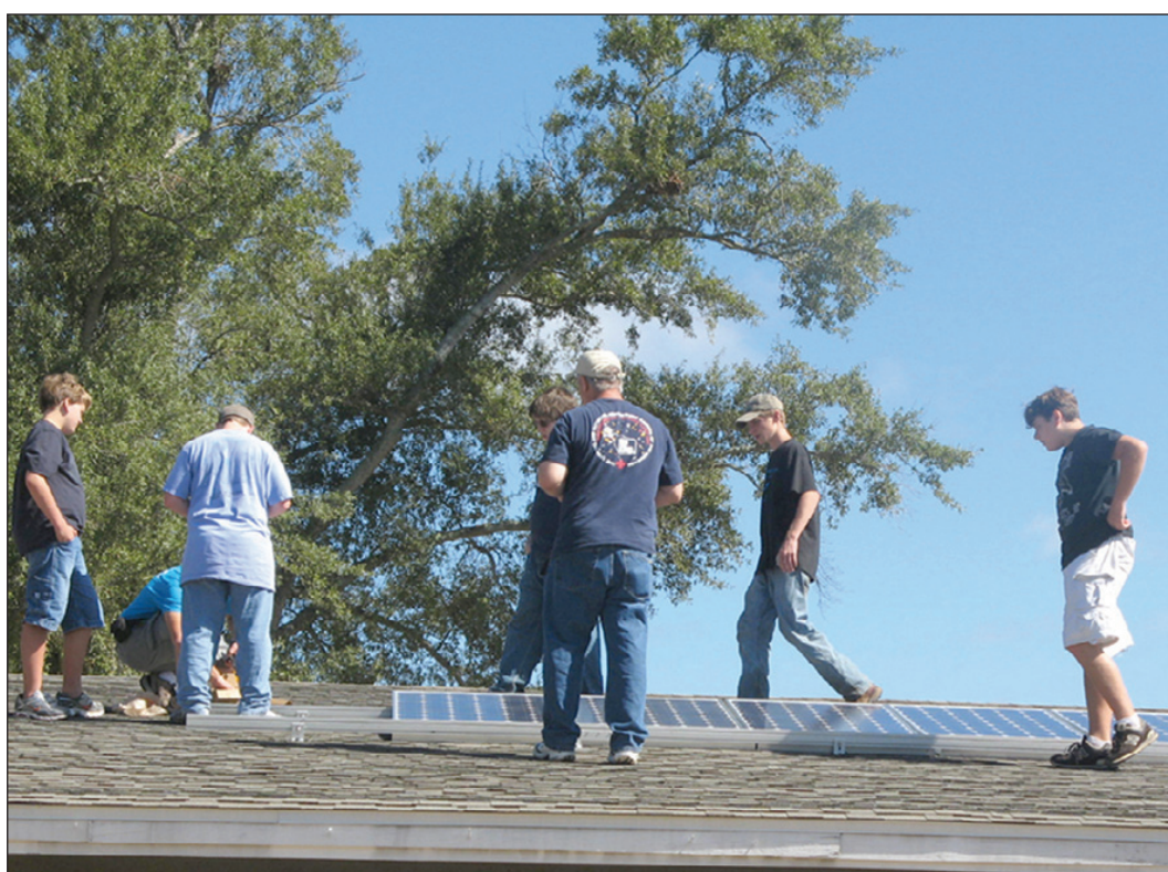
Members of the Science Club of St. Margaret of Scotland Catholic School in Lake Charles, help with the installation of solar panels. The project was the brainchild of St. Margaret graduate Thomas Breaux who came up the idea as part of the process of earning his Eagle Scout award. The school is the first in the State of Louisiana to have solar power. The panels produce twice as much electricity as that needed to operate the school's science classroom and science lab.
