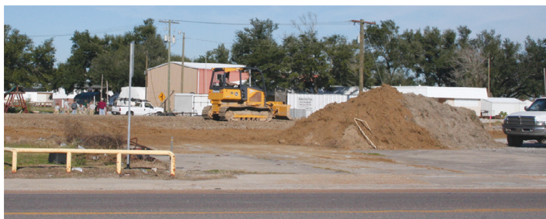
DIRT WORK has begun on the Cameron Food Mart building in Cameron, on the site of the former Gulfway Donut Shop and Mac-Nett buildings. Owners are Orson and Debbie Billings. (Photo by Cyndi Sellers.)
