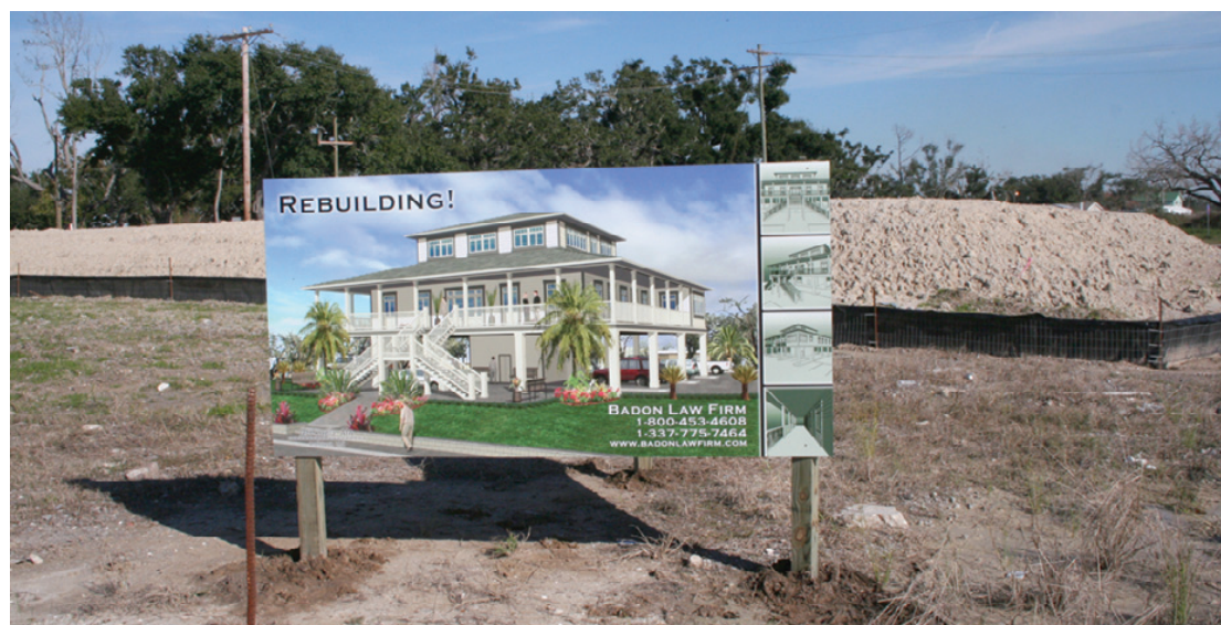
NEW CONSTRUCTION is underway in Cameron. The Badon Law Firm has started work on a new office building near the Court House. (Photo by Cyndi Sellers.)
