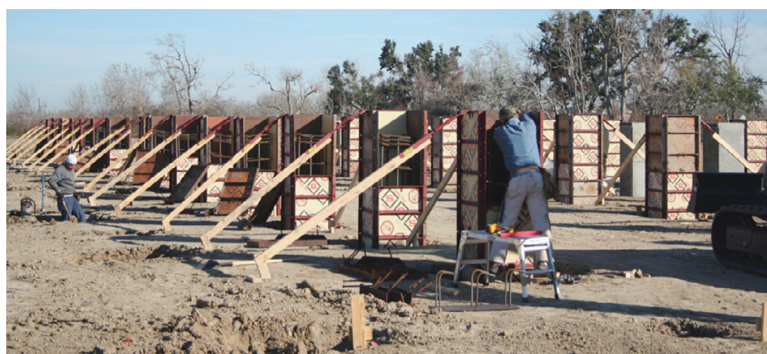
WORKERS FOR Barron Construction Company assemble forms for some of 242 piers that will support the new South Cameron Memorial Hospital. (Photo by Cyndi Sellers.)
