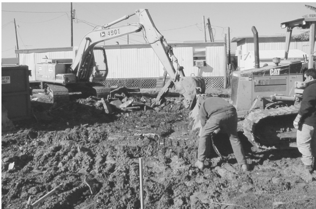
CONTRACTOR WENDELL Wilkerson and his crew are shown cleaning up one of several abandoned houses at Holly Beach. Wilkerson was awarded a $12,800 contract for the project. The cost of the work will be added to the property owner's tax bill and the property will be sold if the bill is not paid. Other property throughout the parish is scheduled for future cleanup.
