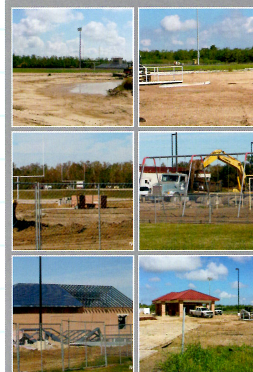
The construction of the football field and track facilities began in the spring of 2013. The facilities were completed in time for the first 2013 varsity football game. These facilities also allowed the track team to have the first meet at home in twenty-eight years.
